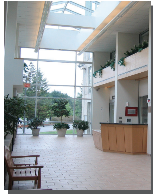
Different environments within Emerson Hospital, such as the Cancer Center above, are easily monitored, controlled and managed—despite each area's very specific HVAC needs.
